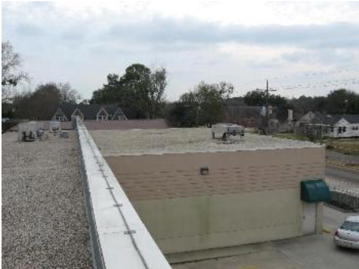
Data Processing Area Overview
