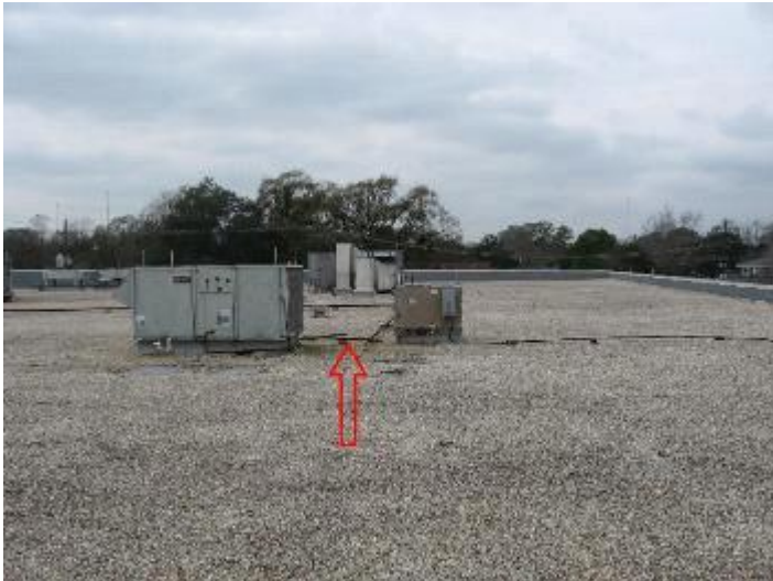
RICOH: Active Leak Area Near front entry over the foyer
