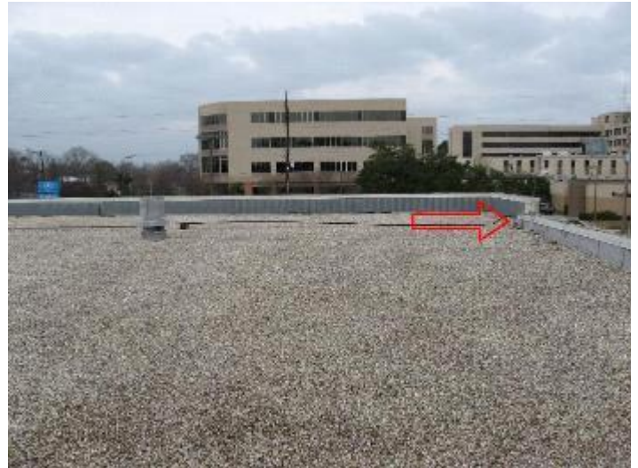
RICOH: Active Leak Area Leak along wall in copy room
