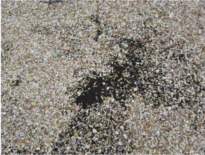
General Conditions Felts exposed
